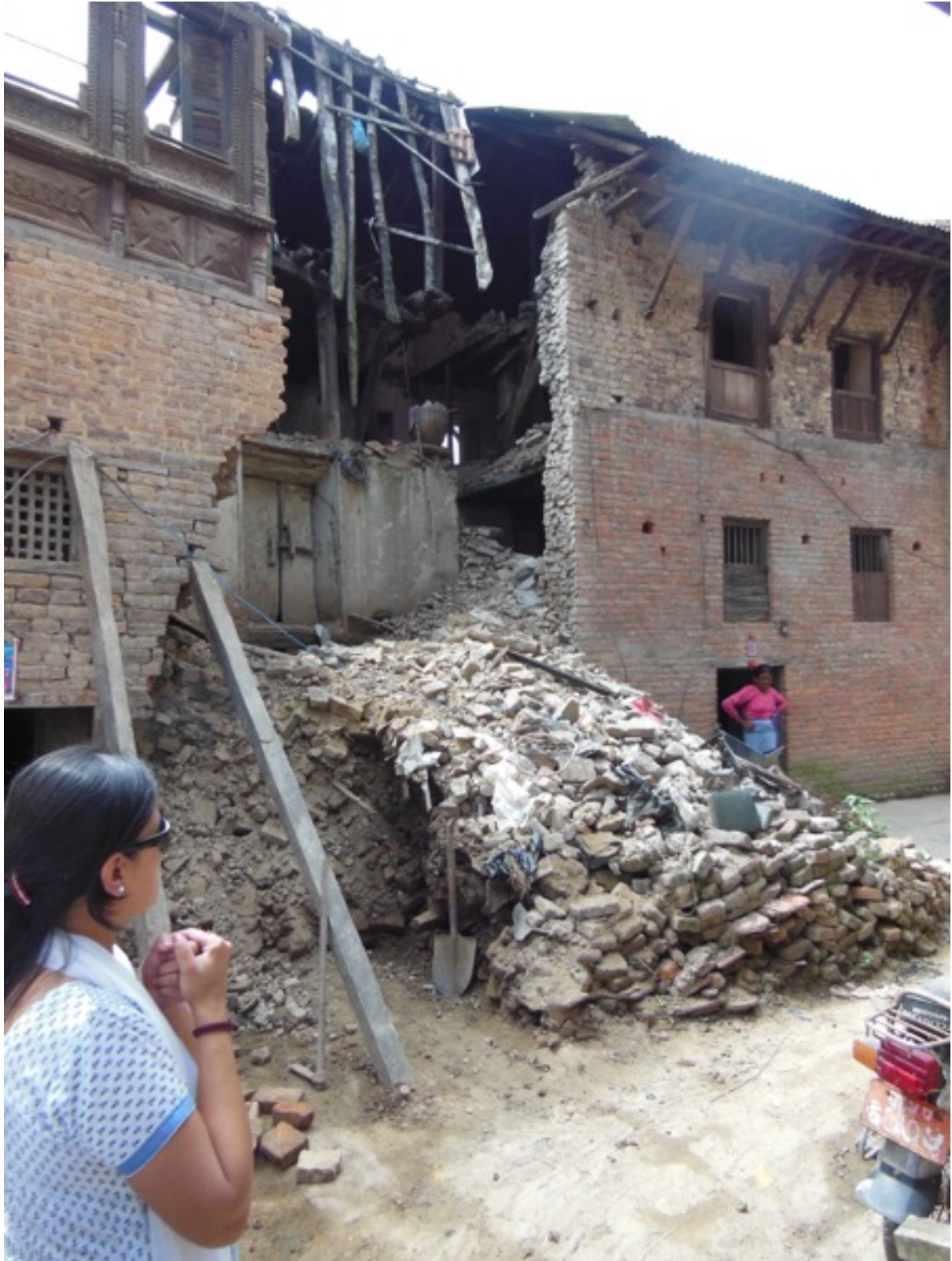
Part of a row of houses. One has almost totally collapsed while next door is still 'habitable'.
